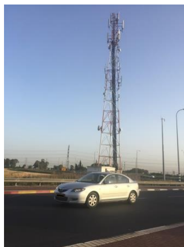
Figure 1. Typical microwave tower (near Hod Hasharon city, Central Israel, 2017). The microwave antennas, the round drum like objects attached to the mast near ground level, are visible.
